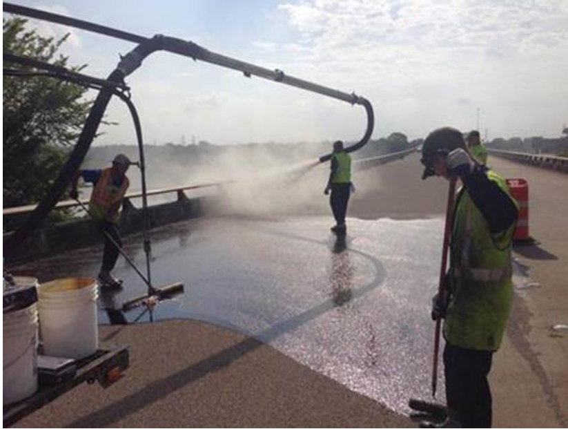
Figure 35. Application of Polymer Overlay Deck Surface Treatment Project (SH 31 WB over Trinity River in the Tyler District).
