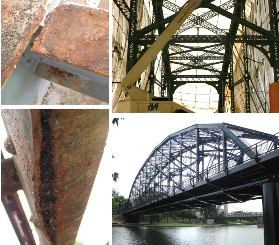
Figure 37. Typical Steel Painting Project, Showing Localized Defects (Left), the Bridge during the Painting (Top Right), and the Bridge after Being Reopened (Bottom Right).
